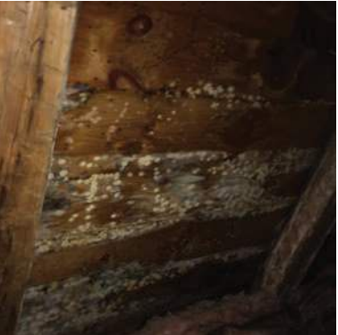
Attic mold, before
